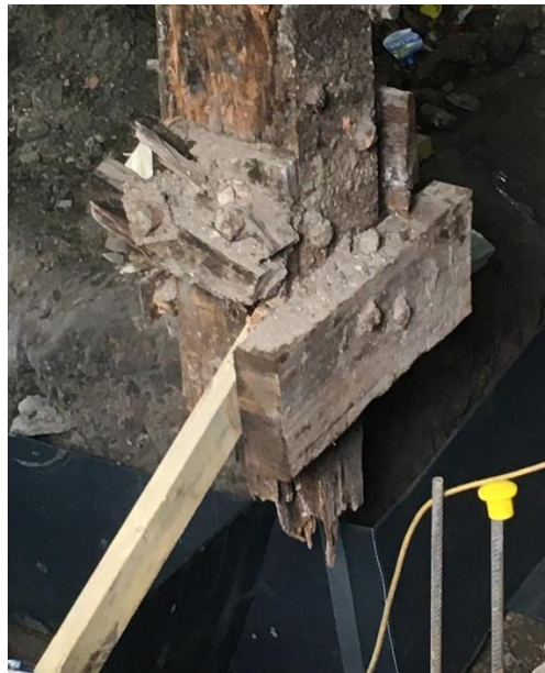
Figure 15. One of the 30 timber piles that support the structure shows extensive rot
